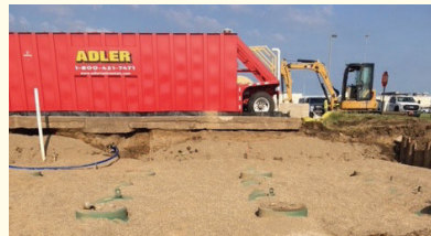
Tank field supplying products to Subaru building.
