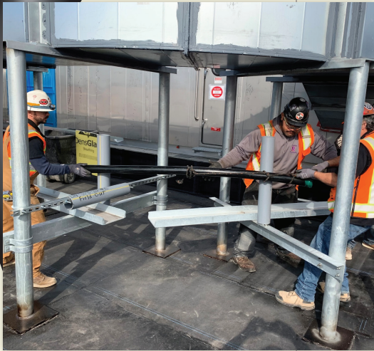
Southland employees pulling the 2" DoubleTrac® piping (UGF-FSP-32) for the fuel oil return line.
