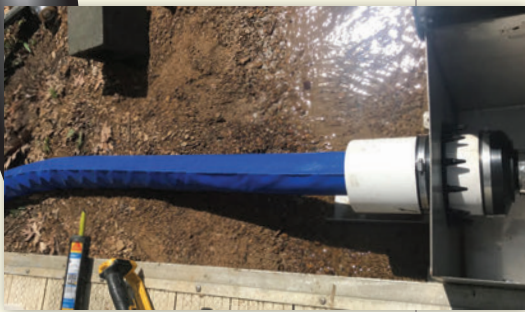
DoubleTrac dock connector from tank to first transition sump.
