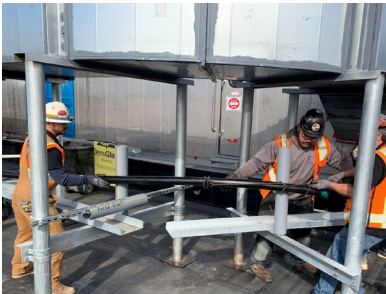
Employees pulling the 2” DoubleTrac® piping (UGF-FSP-32) for the fuel oil return line.
